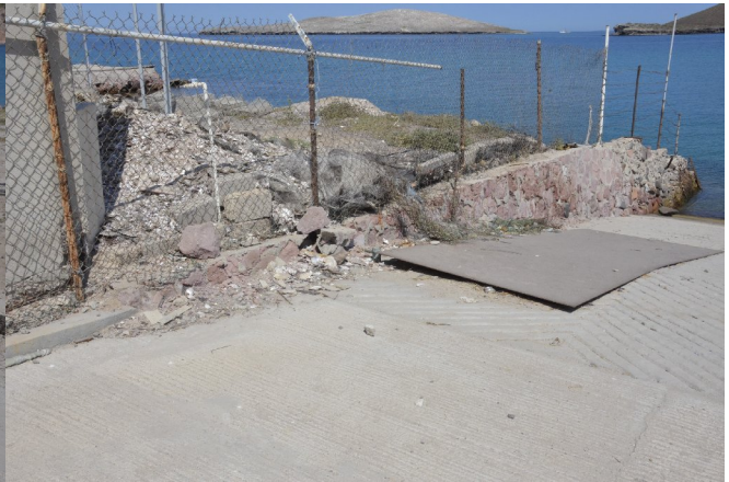
Example of disrepair
