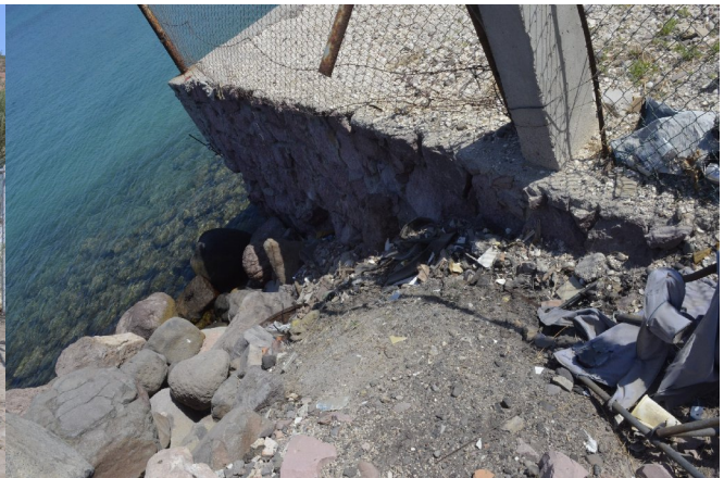
Trash on seawall
